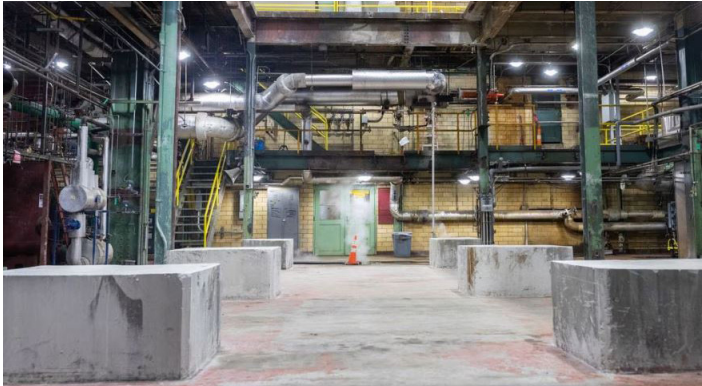
The space where new electric boilers will be installed to help decarbonize Vicinity Energy's heating systems at the Kendall power plant in Cambridge. NATHAN KLIMA FOR THE BOSTON GLOBE
