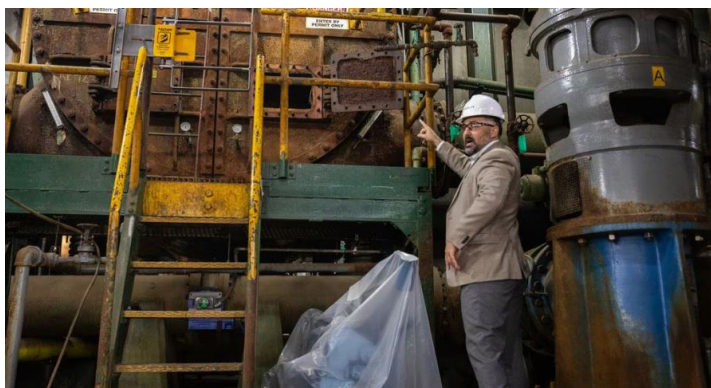
Kevin Hagerty, Deputy CEO and COO at Vicinity Energy, showcases old water pumping infrastructure due to be replaced by new electric boilers at the Kendall power plant in Cambridge, MA. NATHAN KLIMA FOR THE BOSTON GLOBE
