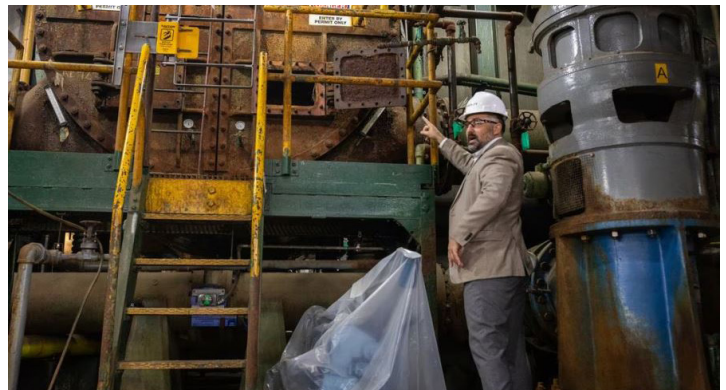
Kevin Hagerty, Deputy CEO and COO at Vicinity Energy, showcases old water pumping infrastructure due to be replaced by new electric boilers at the Kendall power plant in Cambridge, MA. NATHAN KLIMA FOR THE BOSTON GLOBE
