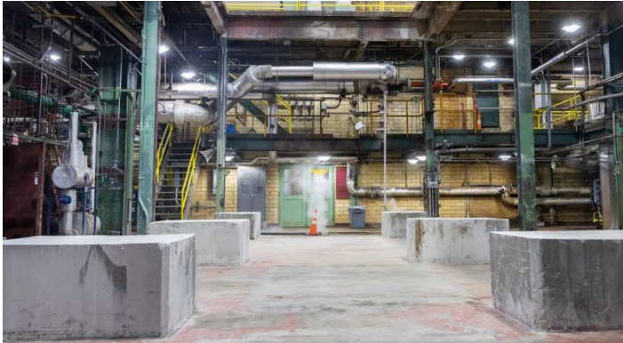
The space where new electric boilers will be installed to help decarbonize Vicinity Energy's heating systems at the Kendall power plant in Cambridge. NATHAN KLIMA FOR THE BOSTON GLOBE
